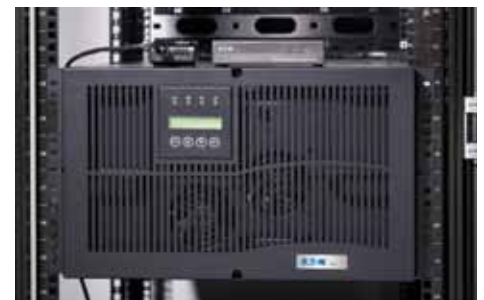
Eaton 9140 UPS with ERM and Environmental Monitoring Probe.
